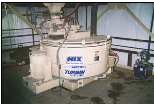
Model 20 TPH Series II DustMASTER installed under truck dump hopper.
