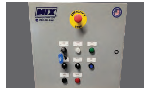
PLC based hoist controls
